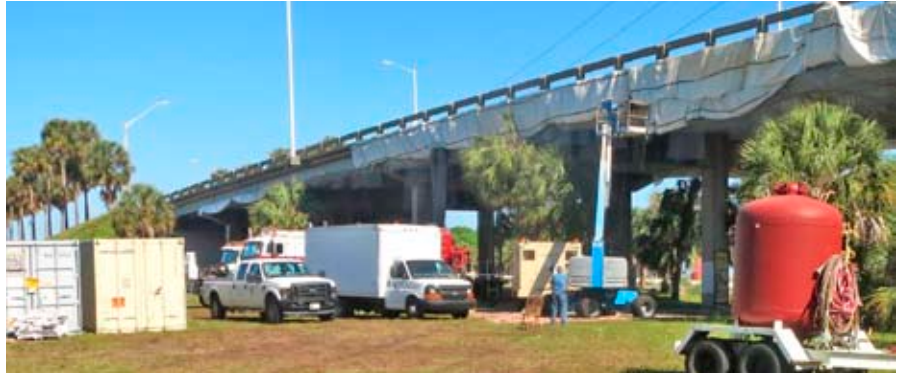
Massive 4 Months of Sandblasting, Priming, Painting the steel beams of Tyrone Overpass.
