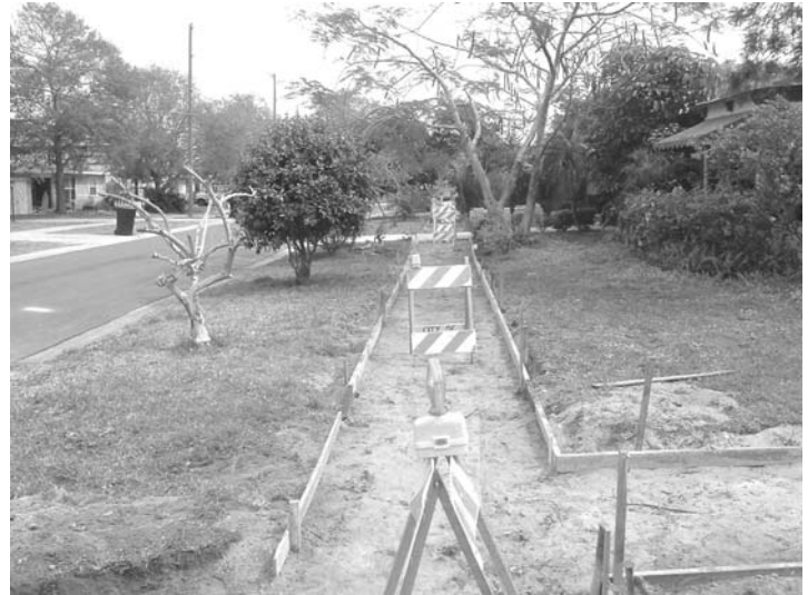
The city installed new sidewalks and repaired broken ones in several locations in our neighborhood.
