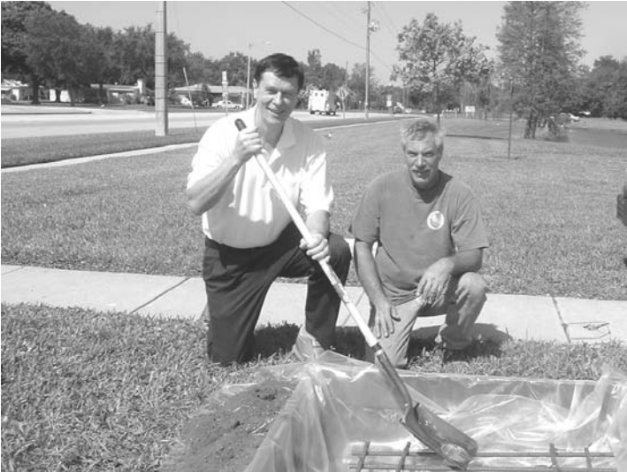
JTCA President Tom Killian and Bill Martin 05 Partnership Grant Builder install rebar for the pouring of the monument pad. Four monuments are being built in our Industrial Park to identify the park.
